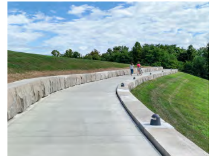
Depending on existing conditions and/or regulatory requirements, trail design can take on different forms. The Silver Creek Trail in New Albany was built on an earthen levee requiring a retaining wall on both sides of the trailway.
